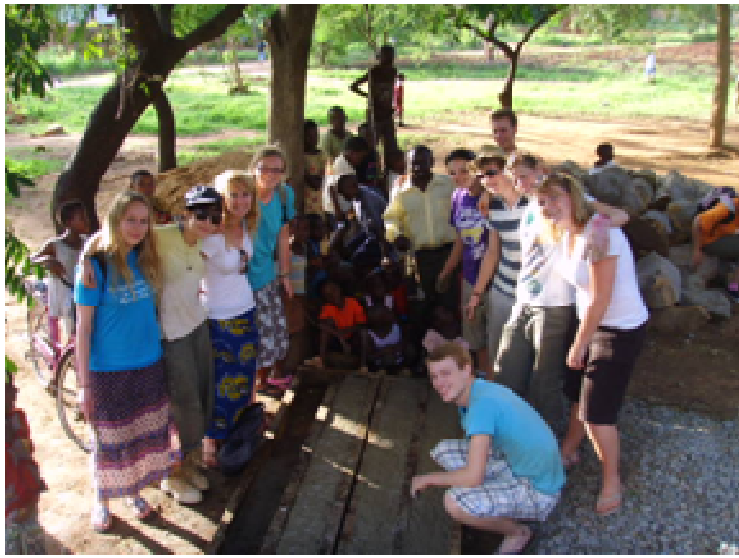
Our team and some villagers after building our first concrete lintel (which makes the base of a toilet)
